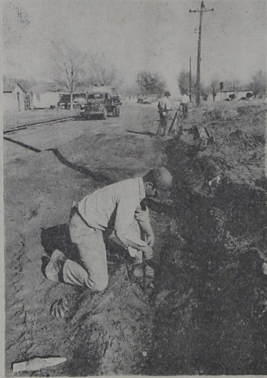
RUNNING LINES on the last 10 blocks of the curb and gutter work of Texico's big paving project is this worker for Thomason Construction Company of Denver City. Forms are placed according to his calculations.
