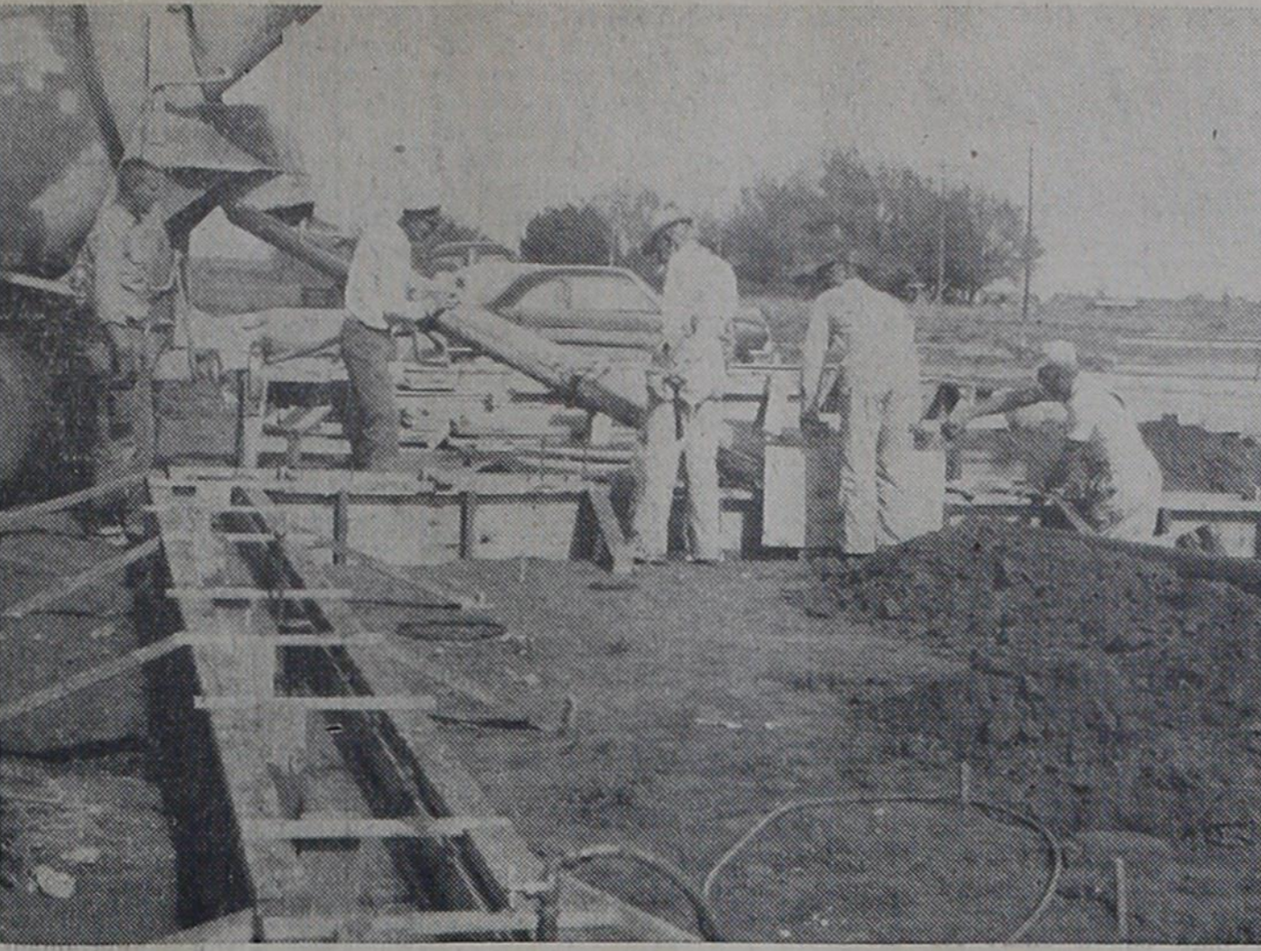
WORKMEN POUR foundations for the new home economics building under construction at Farwell School. Located across the street from the gymnasium, the 40'x72' structure will house a kitchen, living room and dining room area and a small bedroom and bath, as well as a sewing room and grooming center and fitting room. Bill Garrett is contractor for the work.
