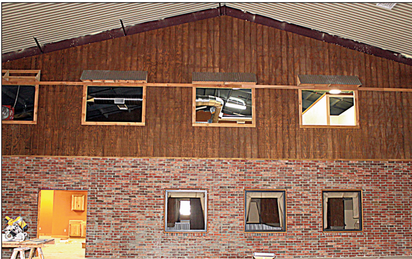
Inside the main meeting room, brick and wood veneer give character to the center. On the second floor, a large coffee room will be a great spot for meeting friends or just enjoying a book.
