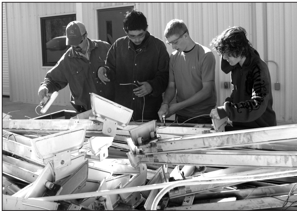
The plumbing, heating, lighting, and other equipment removed from the old cafeteria complex is not being disregarded. From left, instructor Terry Whitener, Miguel Reyna, Gentry Doolittle, and Joseph Jones disassemble and salvage lighting fixtures for FFA chapter projects or for sales to raise chapter funds.
