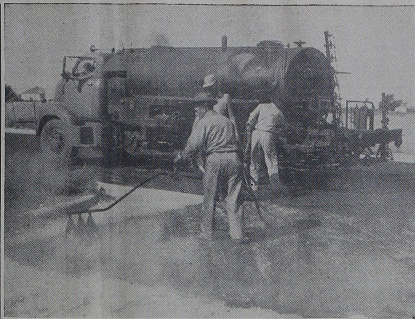
FIRST COAT — Workmen for Capperton and Amerson, paving contractors from Lubbock, begin shooting the asphalt on a First Street intersection Tuesday morning. Work on the four block project is scheduled to be wound up this week.
