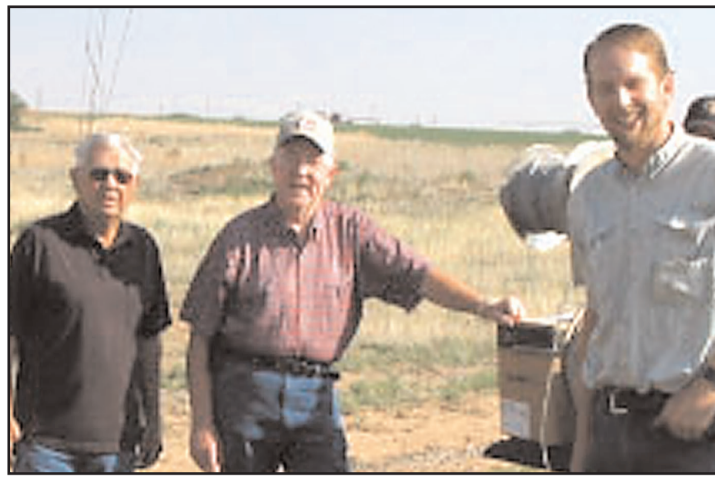
Andy Garza and Jim Bob Swafford assist David Carr of AEI to install wind data equipment. Photos courtesy of BEDC.
