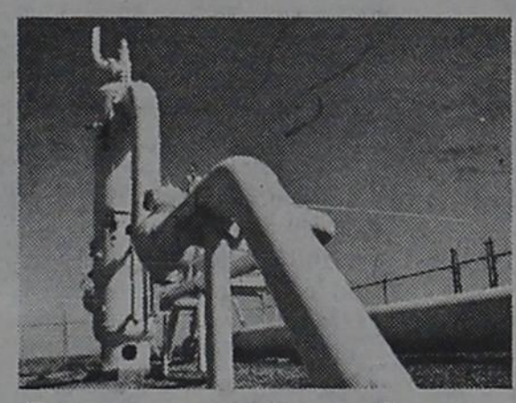
So was natural gas.
