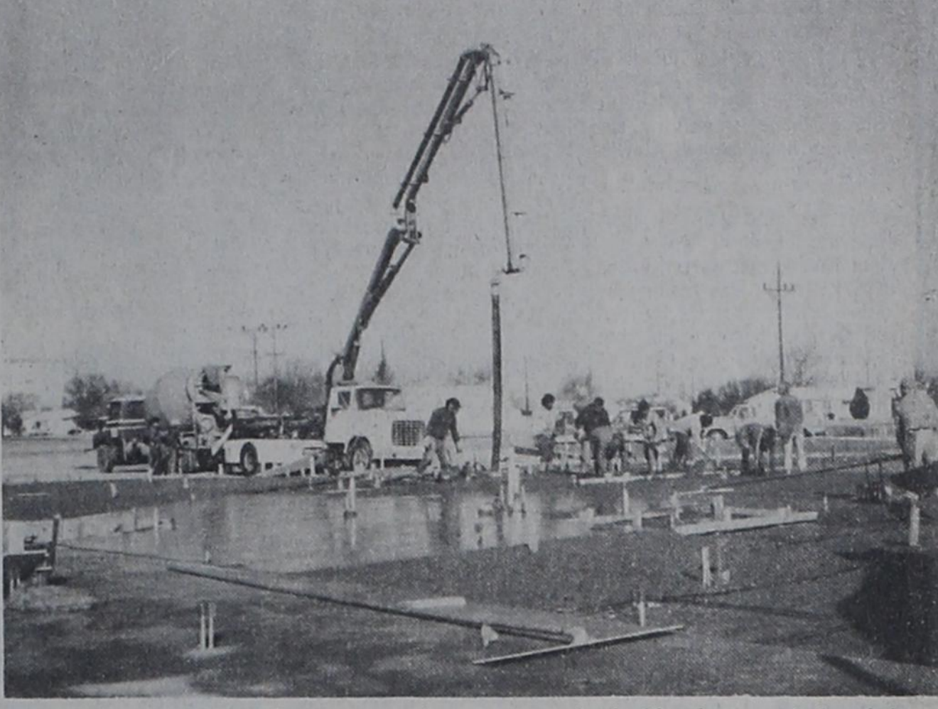
STRANGE ANIMAL - What appears to be a strange animal with a long, crooked neck is actually a device which workmen were using last week to pour concrete for the foundation of the Farwell Nursing Home. The device was used to pour areas which the regular concrete trucks could not reach. Work on the 100-bed nursing home began Monday, Jan. 12, and is to be completed in 165 calendar working days at a cost of $560,000.
