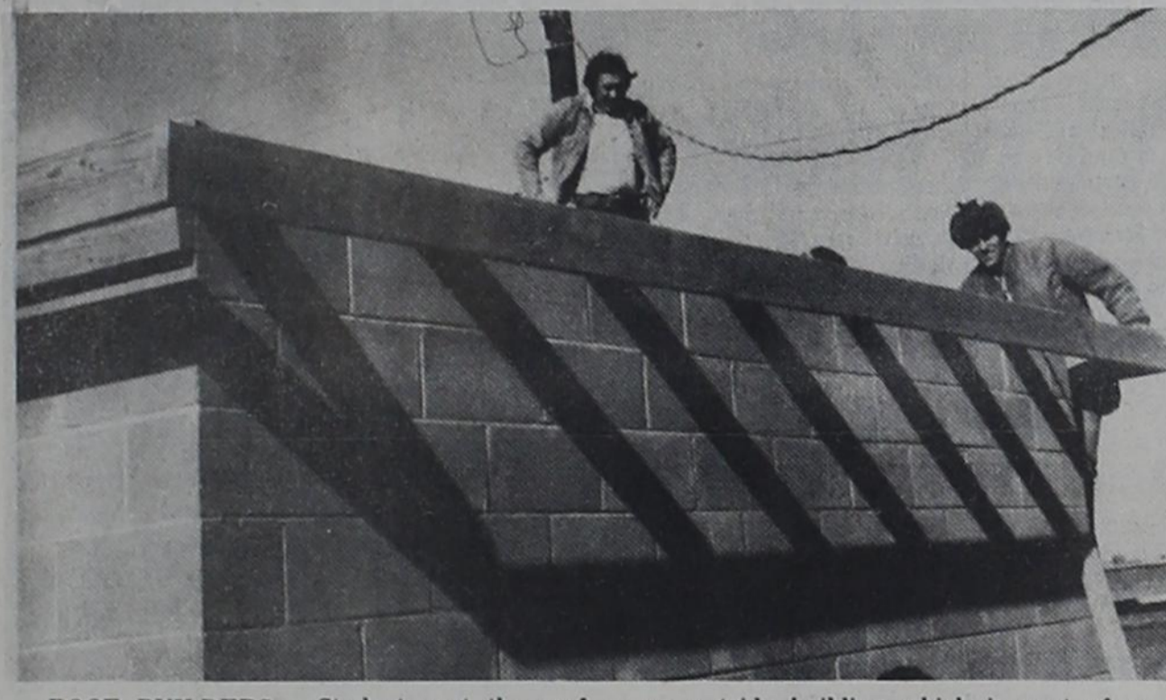
ROOF BUILDERS - Students put the roof on an outside building which is part of a residence constructed by the High Plains Area Vocational Technical School at 1308 Lexington Road in Clovis. Shown are Tony Baldo, left, and John Chavez.
