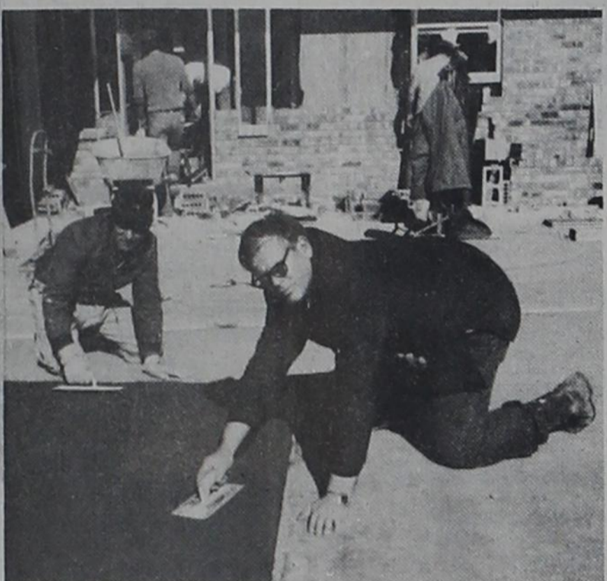
SMOOTH WORK - Students, Bob Hester, left, and Claude Willette, finish concrete in front of a new home which was constructed by persons enrolled in programs at the High Plains Area Vocational-Technical School in Clovis.
