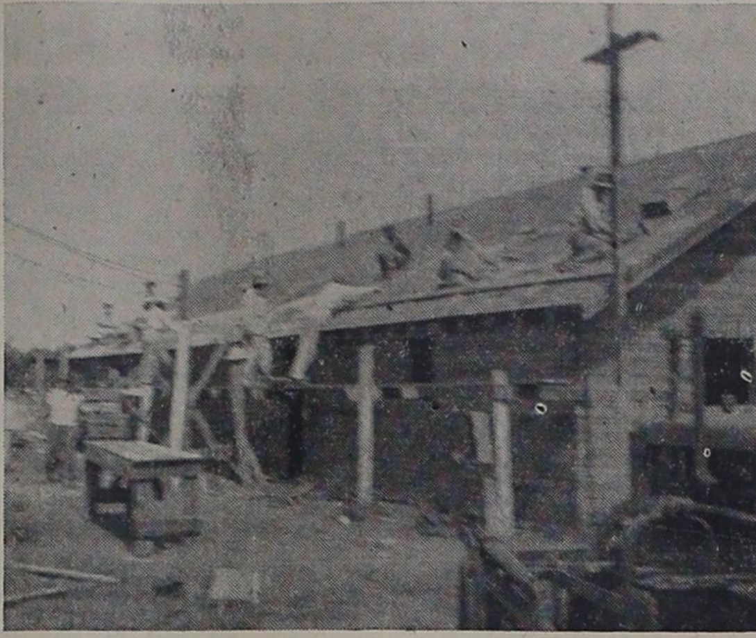
Five men attack the Field House roof. It was this kind of voluntary cooperation which made possible the rapid completion of the Farwell school project.
