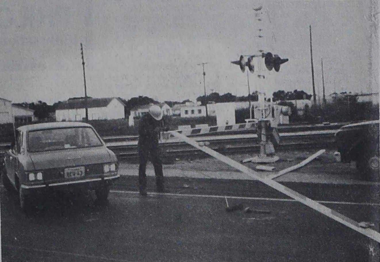
OOPS, AGAIN - Dwayne Williams, signal maintenance worker for Santa Fe Railway, was out Friday evening, Aug. 22, doing repair work on the crossing arms installed on the main street joining Texico and Farwell. Someone was involved in a "hit and run" situation involving one of the arms. Williams, who resides in Texico, reports that the arms cost approximately $300 each and this is the sixth such incident to occur since the installation of the arms. The car shown in the picture was not the culprit, but belongs to Williams.
