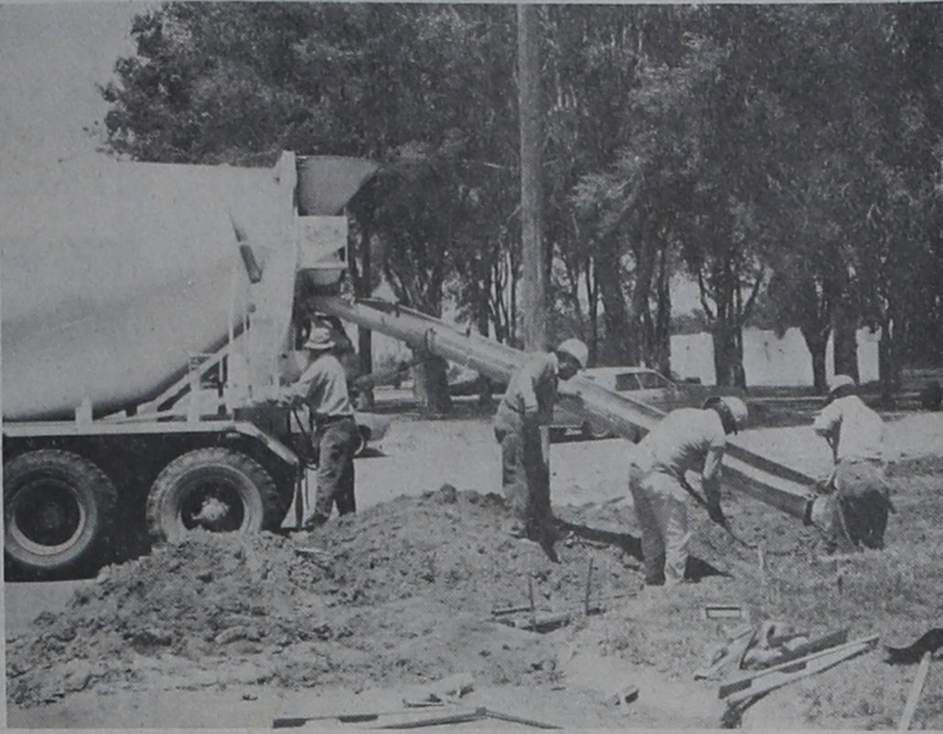
CURBS LAID - Construction of the parking lot at the Parmer County Courthouse continued this week as workmen poured the concrete curbs for the parking area. Shortly after the noon hour Tuesday, concrete was poured and curbs were shaped, with more than half the curbing for the area south of the courthouse completed by the end of the day.
