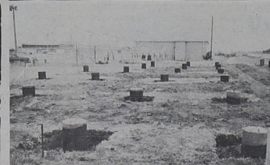
section of bleachers to be constructed at the football field. Construction and renovations at the local school are being financed by the sale of bonds authorized by voters during a bond election conducted earlier during the 1974-75 year.
