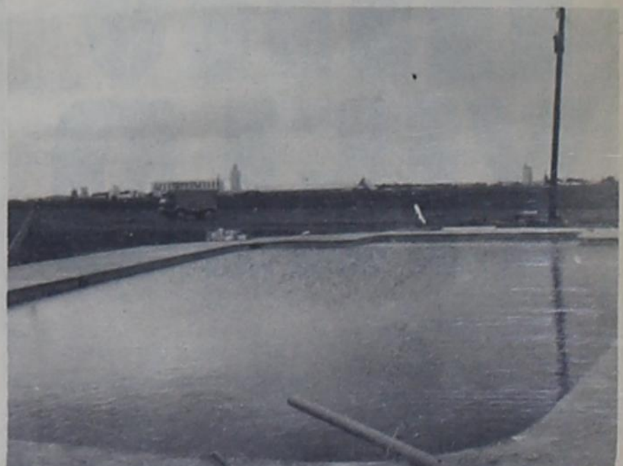
ALMOST READY -- The swimming pool at the Farwell Country Club and the bathhouse facilities should be completed by the end of next week, according to Bill Prince, chairman of the planning committee. However, the pool will not be opened until a qualified lifeguard can be secured. The pool has already been filled with water and the chlorinators will be put into operation within the next few days.
