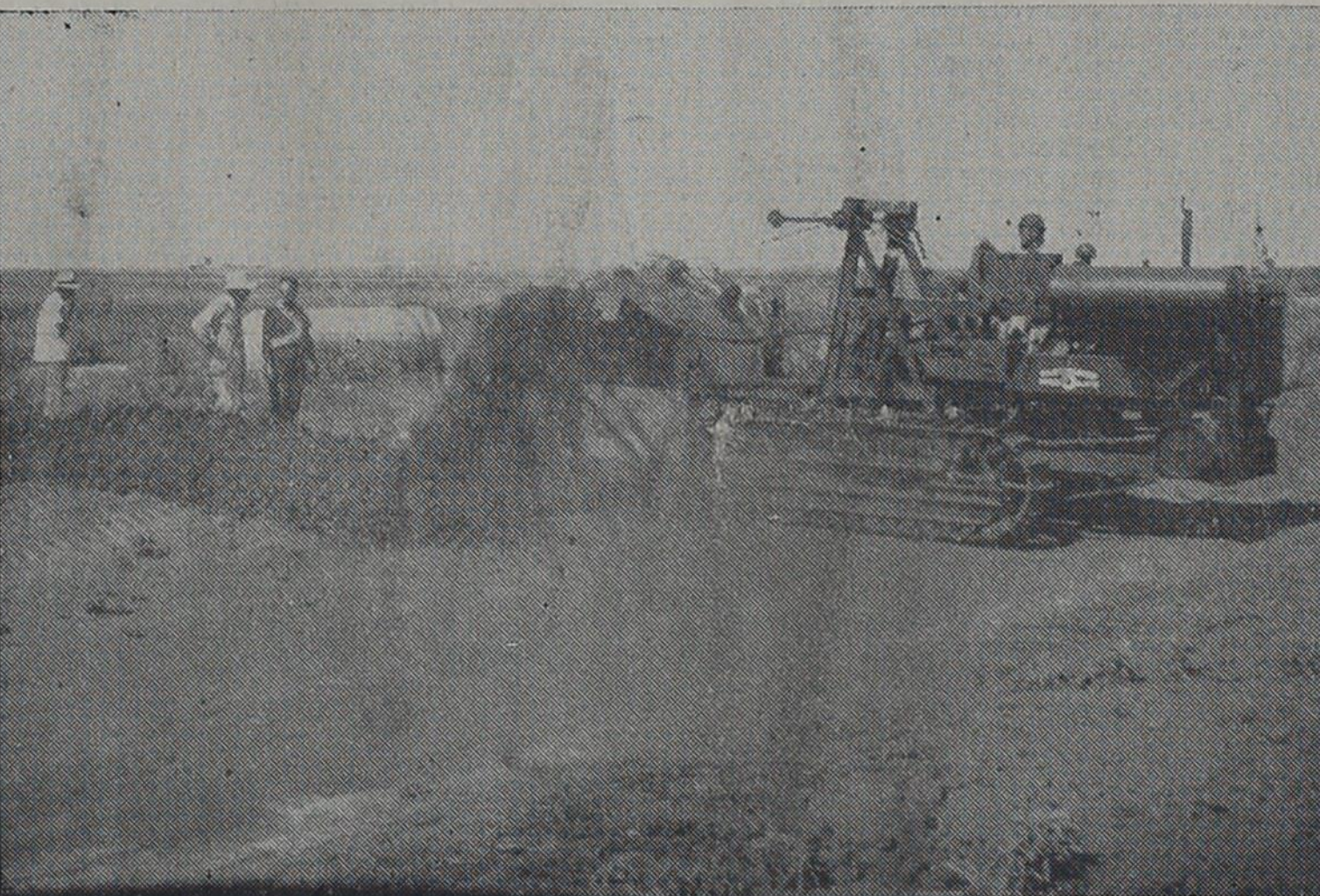
BEATS DIGGIN' BY HAND —This ditch digging machine eats up the dirt on the D. J. Brown farm as installation of the natural gas line southwest of Texico gets underway. Looking on are Elmer Riley, far left, Brown, center, and Travis Binion. Riley and Binion are of B and R Construction Company, Lubbock.
