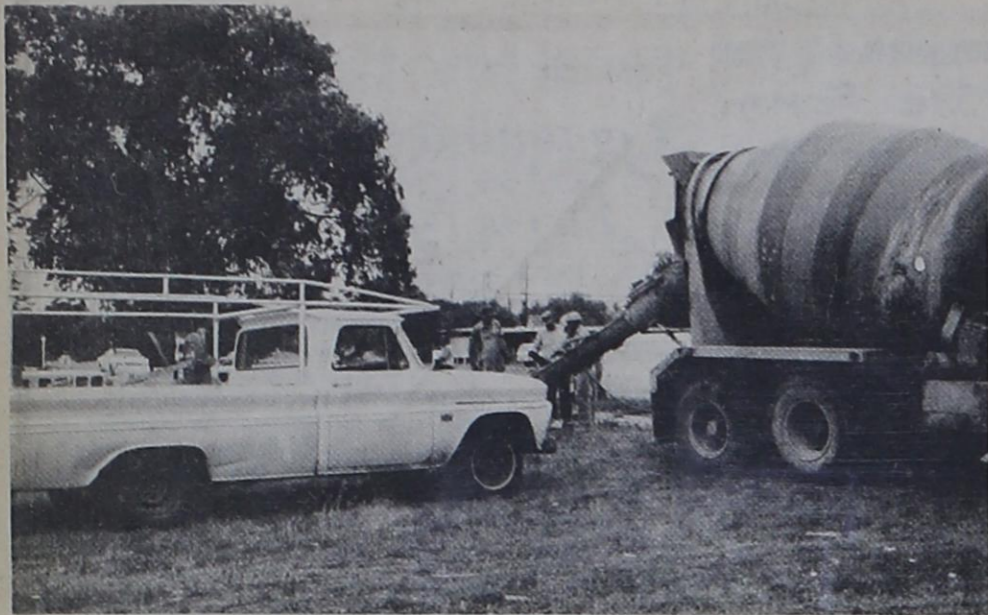
FHA OFFICE BUILDING STARTED - Nance Construction Co. began work this week on an office building which will be located across the street north from Aldridge, Harding and Aycock law offices. The new offices will house the Parmer County office of Farmers Home Administration. Concrete has been poured for the foundation and cement blocks have been unloaded at the site in preparation for the construction.
