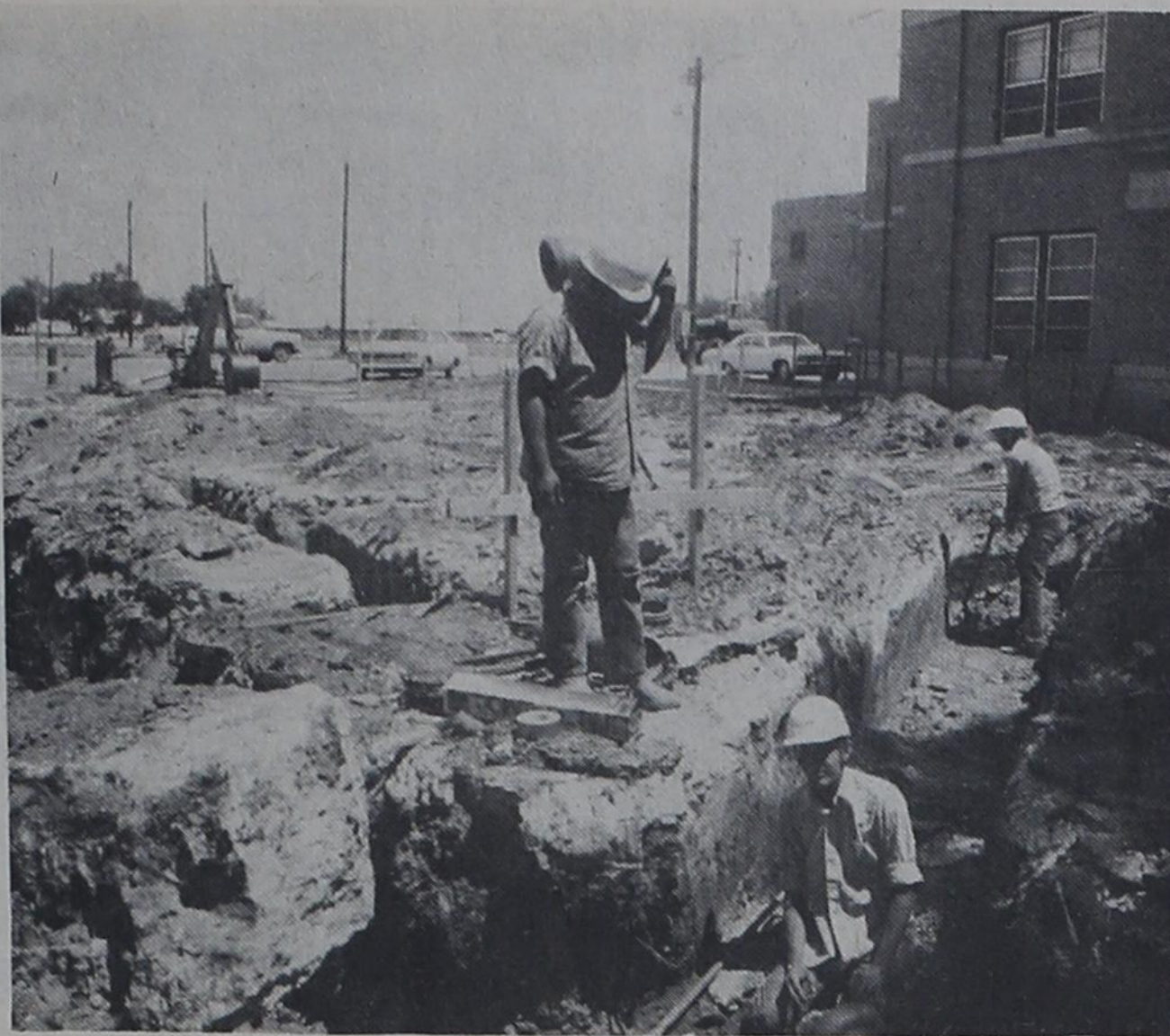
CONSTRUCTION PROGRESSES - Construction is progressing on the Parmer County Law Enforcement Center as workers excavate in preparation to lay sewer lines. Working on the project are Denny Busbea, front; Ruben Valdez, left, and Frank Cocke, all of Lubbock.
