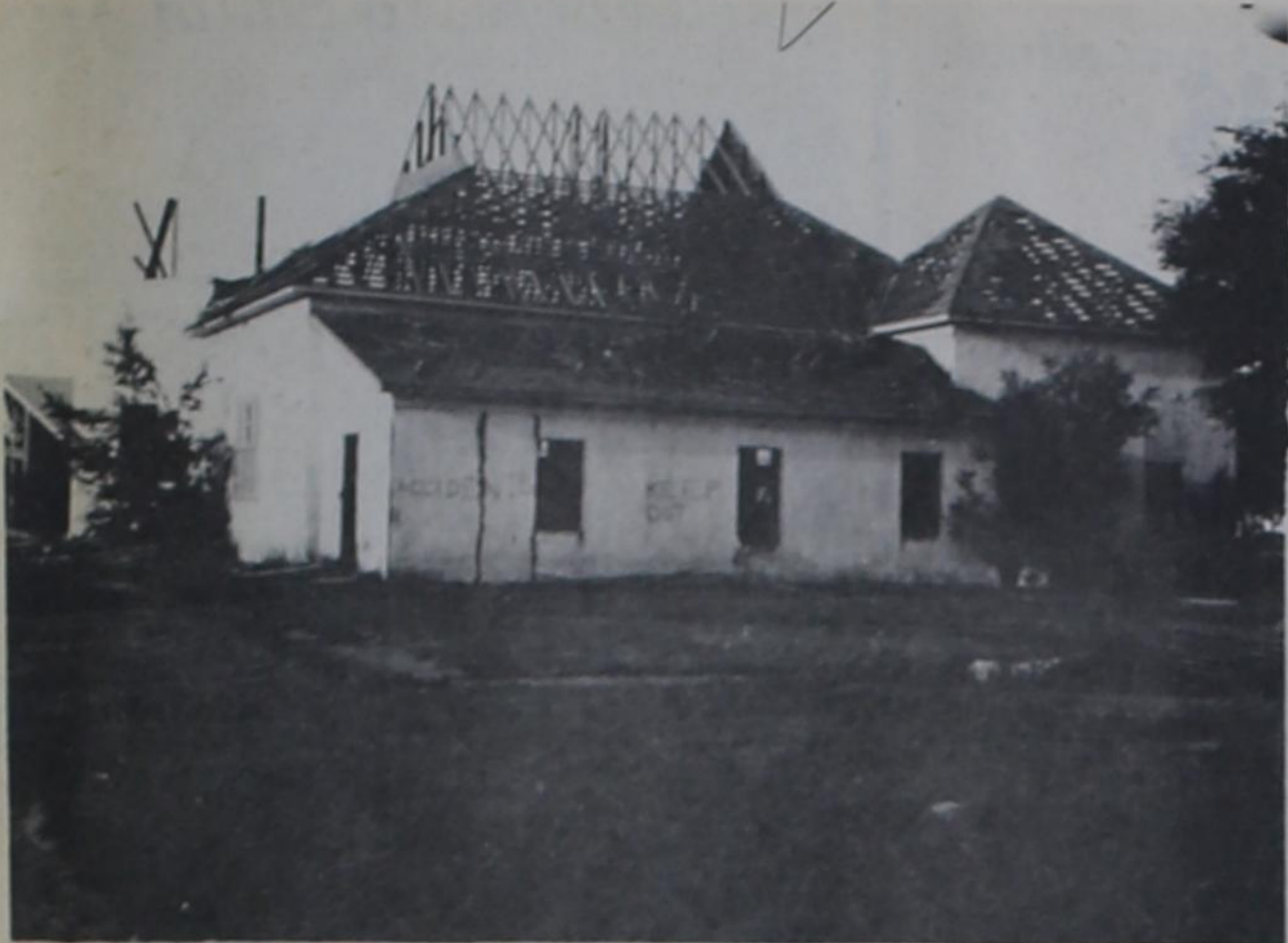
END OF A LANDMARK - With the removal of this 66-year-old building, a landmark has been erased. The building was erected in 1907 as the home of the newly organized First
