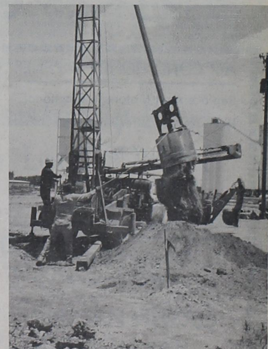
CONSTRUCTION STARTED—This machine was drilling holes called boot pits last Friday for elevator legs for the new Kelly Green Seed Co. elevator which will be in operation by August, according to J. W. "Pat" Patrick, manager and co-owner. Kelly Green elevator was destroyed January 24 by fire apparently touched off by a dust explosion.
