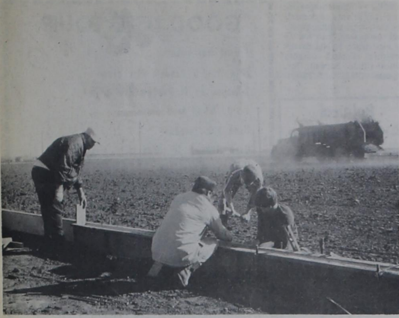
MAKING PROGRESS -- Volunteer muscle power is making possible the construction of a cinder track for use by Farwell Schools. James Craig, Farwell Junior High principal, left; Harry Sheets, project engineer, kneeling; Mark Haseloff, hammering; and Thad Phillips spent some time Monday afternoon rimming the track while fertilizer was dispensed on the inside of the track by the truck in the background. Several students, townspeople and farmers have lent equipment and labor to the project. Joe Jones reports that $3675 has been collected to date to pay for the track, but he reminds interested persons there is still time to help either by providing muscle power or donating to the project.
