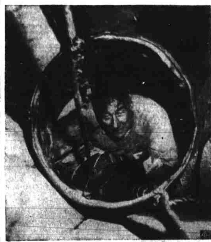
TRAPPED IN 20-FOOT SHAFT—Dominick Atteo, 45, is trapped in a 20-foot well that collapsed while being dug under a Brooklyn garage. Fully conscious he directs rescue workers as he guides a pall full of dirt to the surface. An oil drum, its ends knocked out, has been slipped in place to form a protective barrier. (AP Wirephoto).
