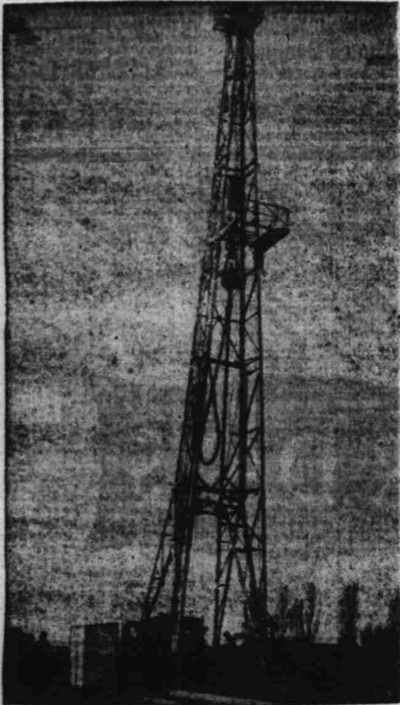
OIL FOR THE LAMPS OF LONDON — A 65-foot derrick drills for oil in the center of Gibbon's Road, a recreation ground, at Willemsen, London, England, as work is started by the D'Arcy Exploration Co., which hopes to tap a huge reservoir of oil 2,200-feet beneath the earth's surface. (AP Photo).
