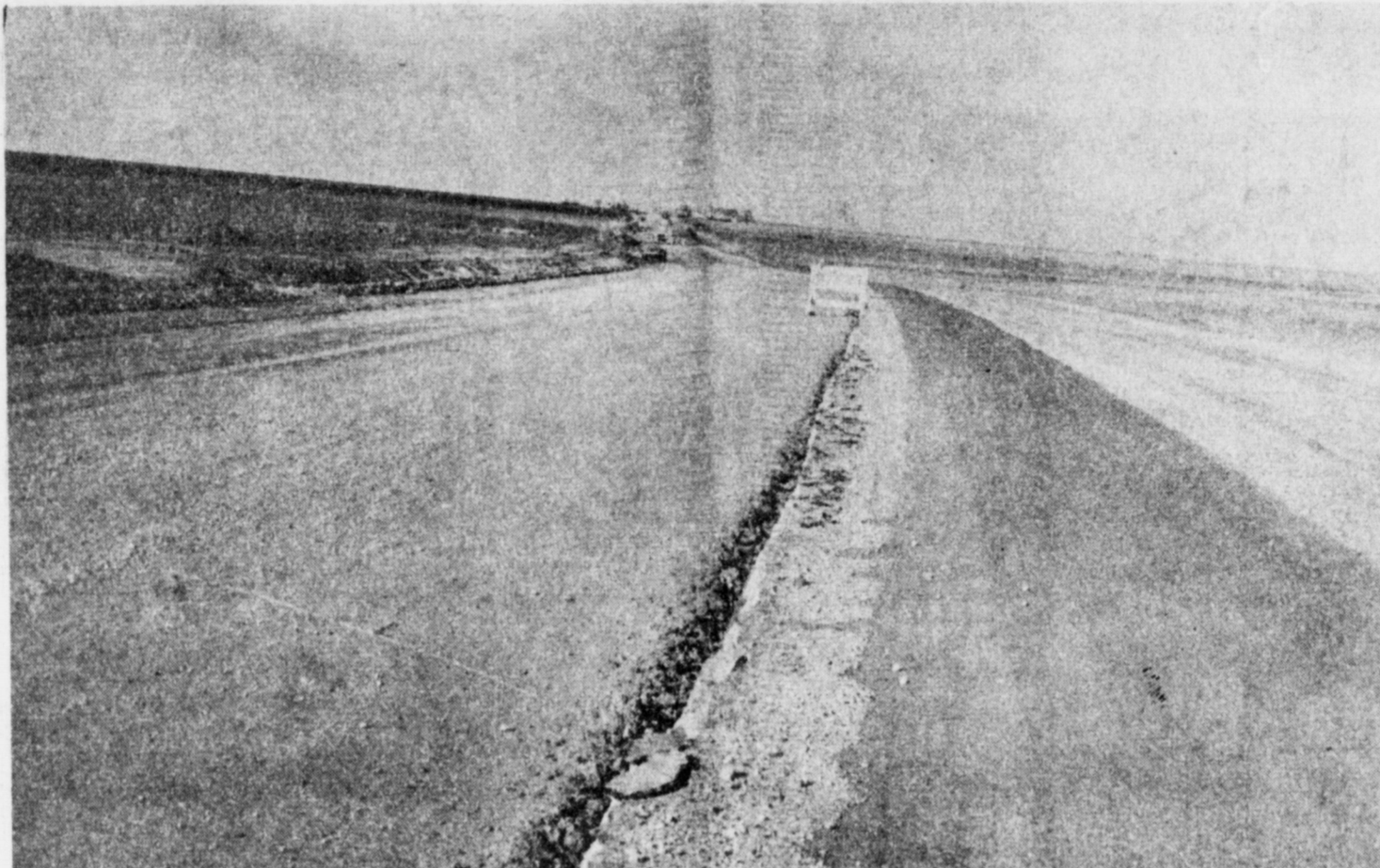
ROAD CONSTRUCTION . . . Motorists traveling from Muleshoe to Friona can expect to drive on some tore up roads. During the process of widening Highway 214, construction workers have the highway in quite a mess. This drop-off just beyond
