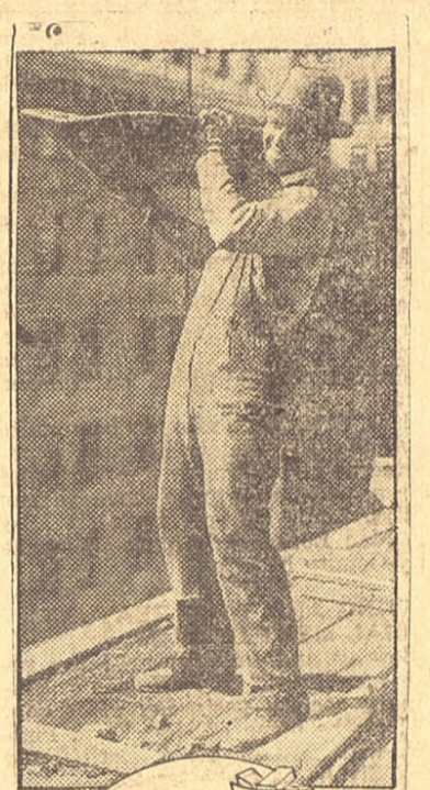
Jerome Brady, Columbia University football star, is discovered laying bricks atop a New York skyscraper to keep in condition. Jerry is a member in good standing of the bricklayers' union.
