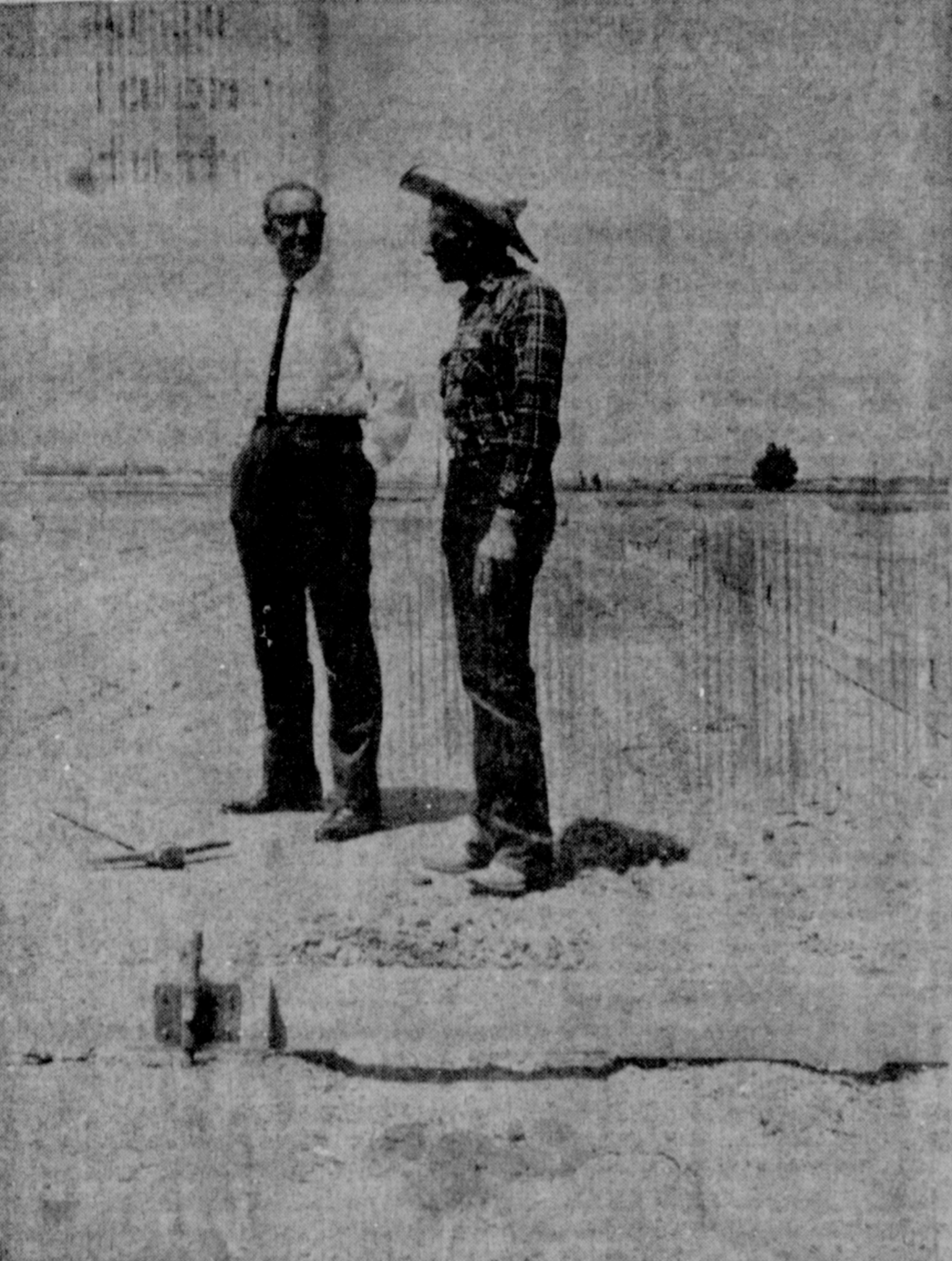
INVESTMENT IN MULESHOE'S FUTURE — Workers this week began erecting foundation forms for the new $100,000 Johnson Furniture Building to be located east of Francis Implement on the Clovis Highway. To have more than 14,000 sq. ft. of floor space, the building will allow Johnson to offer the Muleshoe Trade area a complete selection of furniture. To be of concrete block construction, the building will have a brick front. It is being constructed by B & C Builders of Muleshoe. Here Red Johnson and David Headlee discuss the foundations.
