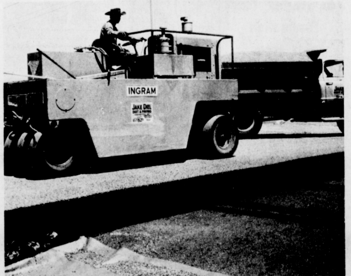
PAVING AND PATCHING FOR PROGRESS--Workmen have been busy patching and repairing city streets while doing extensive paving in other areas of Muleshoe. Much work is being carried out throughout the city with some previously unpaved streets being smoothed and paved for the first time.
