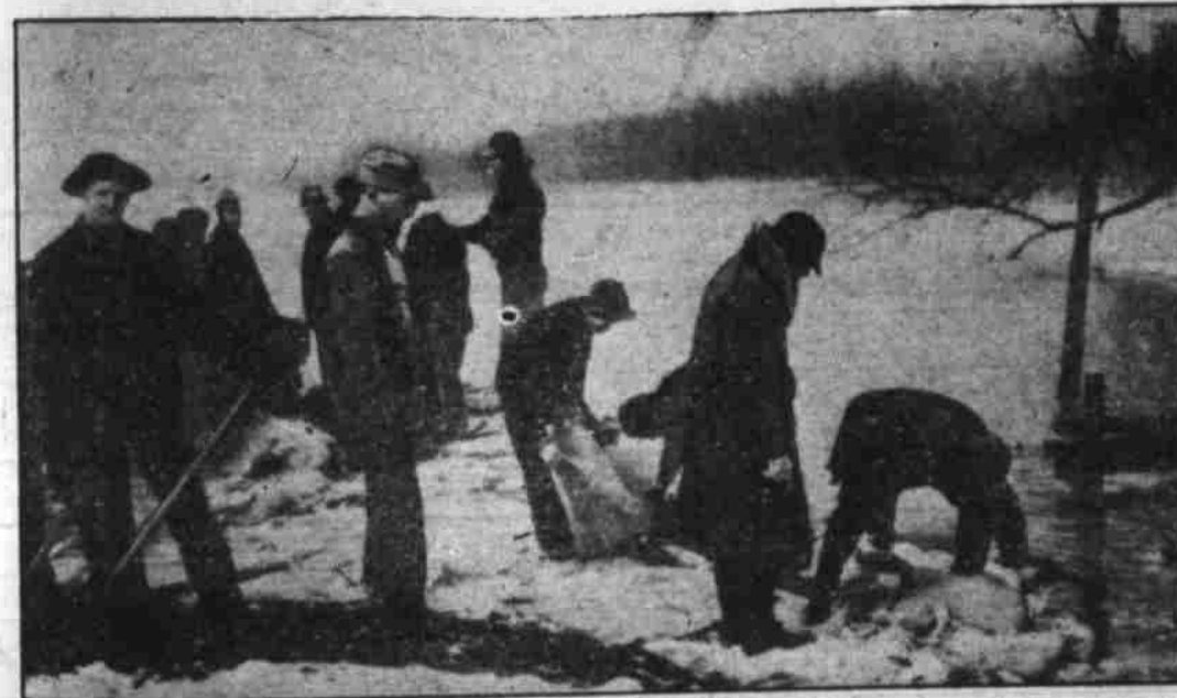
Men and boys are shown working side by side at Wolf Island, in the Birds Point—New Madrid (Missouri) floodway, at the apparently futile task of strengthening the levee enough to hold back the flood waters of the swollen Mississippi. (Associated Press Photo)
