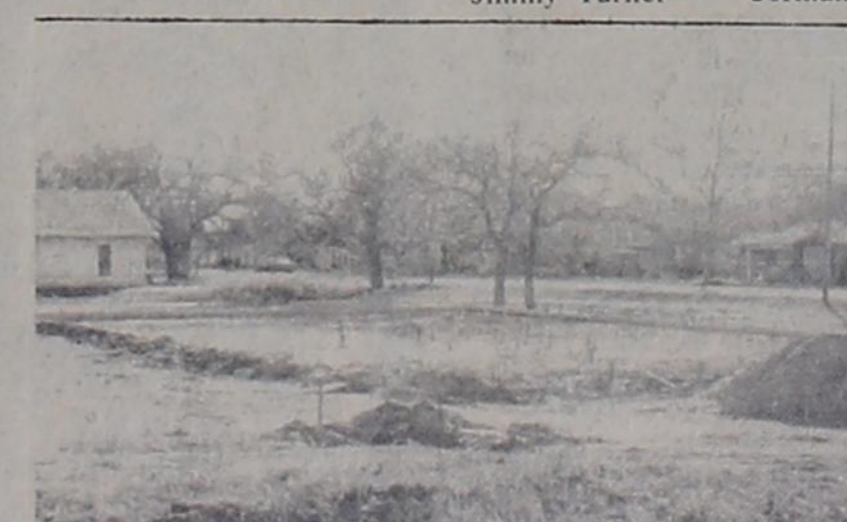
FOUNDATION LAID — Show above is the foundation for the new Texas Federal Inspection Building being built close to Downtown. The plumbing and ground is ready to permit the pouring of the slab.
