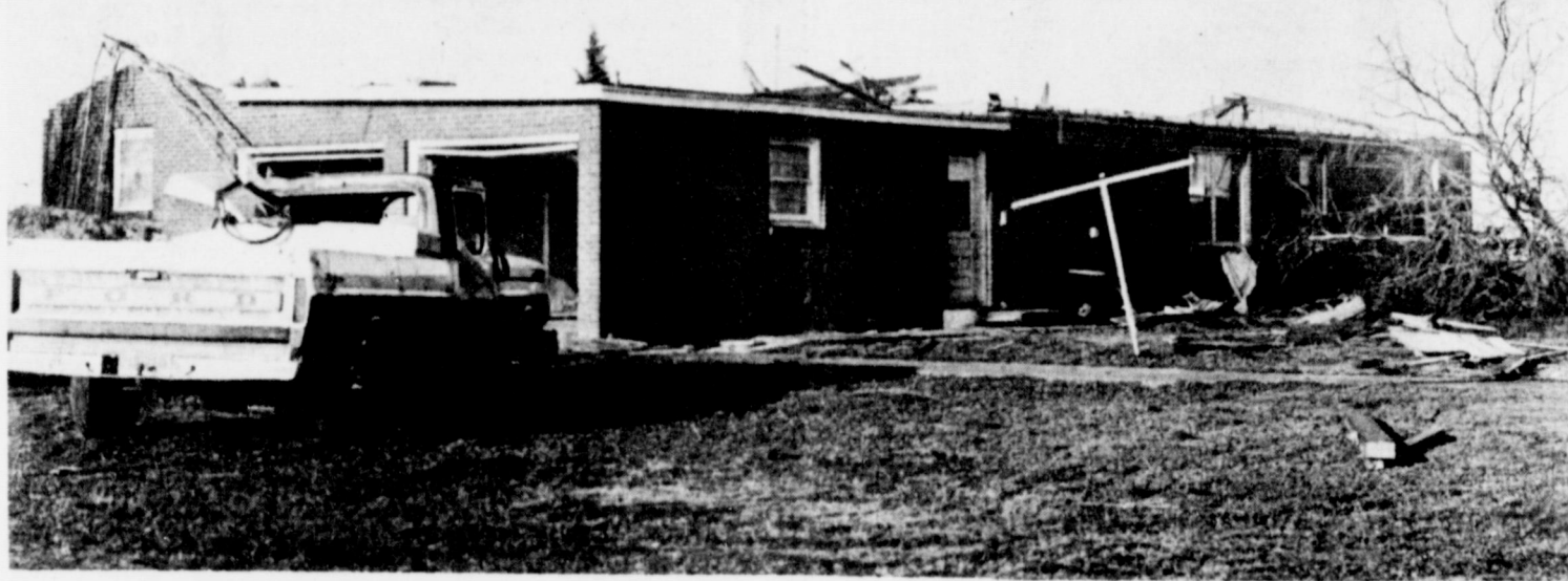
TORNADO CLAIMED VICTIM IN THIS HOME--Mrs. Alton Morris, around 51, was killed Friday night in a tornado near Lazbuddie which unroofed and destroyed this farm home. Debris and litter mark the path of the tornado, which also
