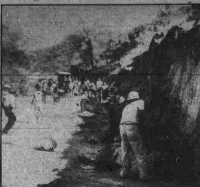
Italian road builders shown creating a military highway leading to the Ethiopian frontier, for use of supply trains carrying food and ammunition from Eritrea to Il Duce's armies within Haile Selassie's country. (Associated Press-Paramount News Photo)
