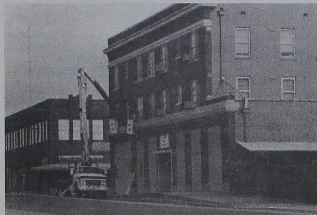
WINDOW CONSTRUCTION — New facial construction is being added to the Gorman Hotel Apartment building. The construction consist of new Storm Windows on the outside of the building. There is also construction being done at Love Acres and Brandon Place.
