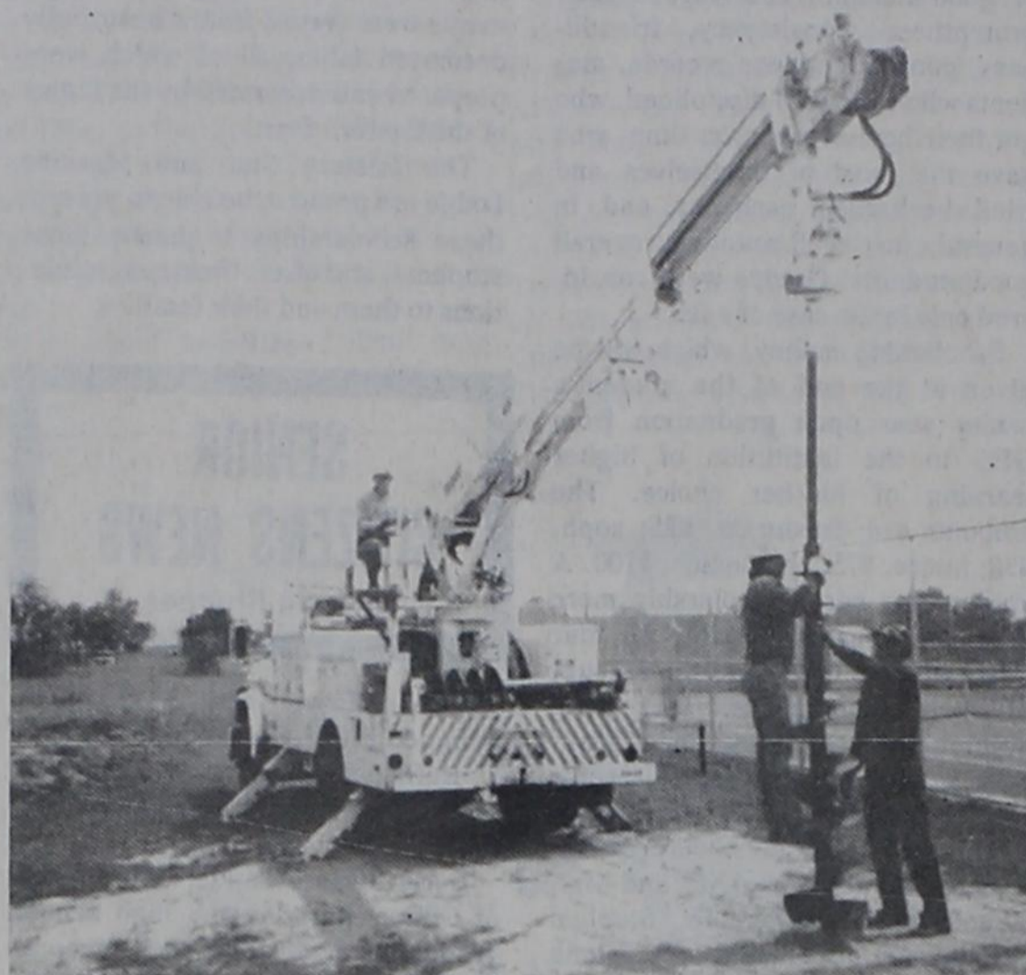
PREPARING FOR NEW LIGHTS — The Tennis Courts in Gorman will soon have lighting thanks to the help from TU Electric truck and two of their employees and Jack Harrison shown above setting the location for the first pole for the new lights.
