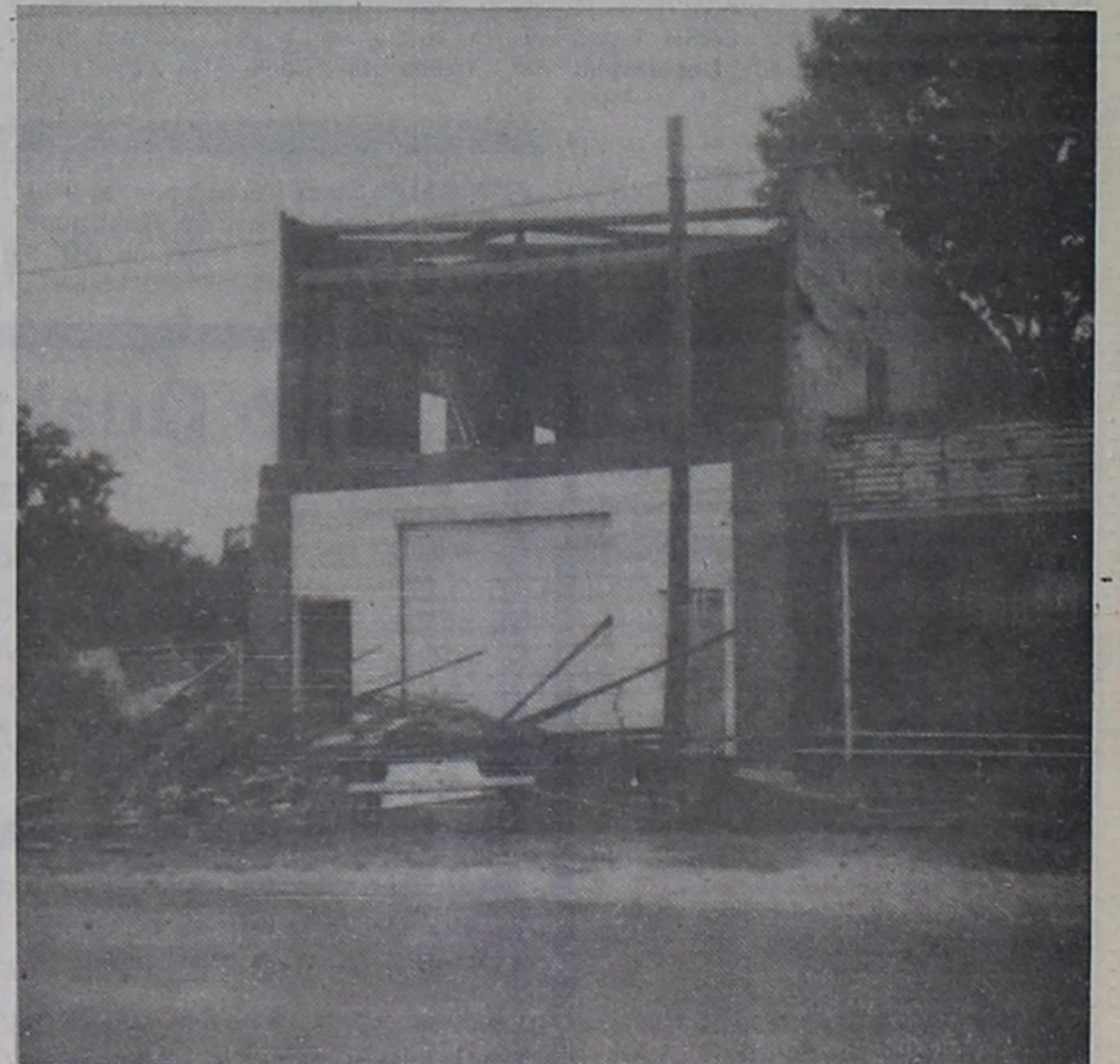
The building on the Corner of Smith Bros. Chevrolet lot is being demolished. The building has been around for a very long time. It is the former E. T. Jones Grocery Store, when many school children bought their candy and school supplies in the 30's.
