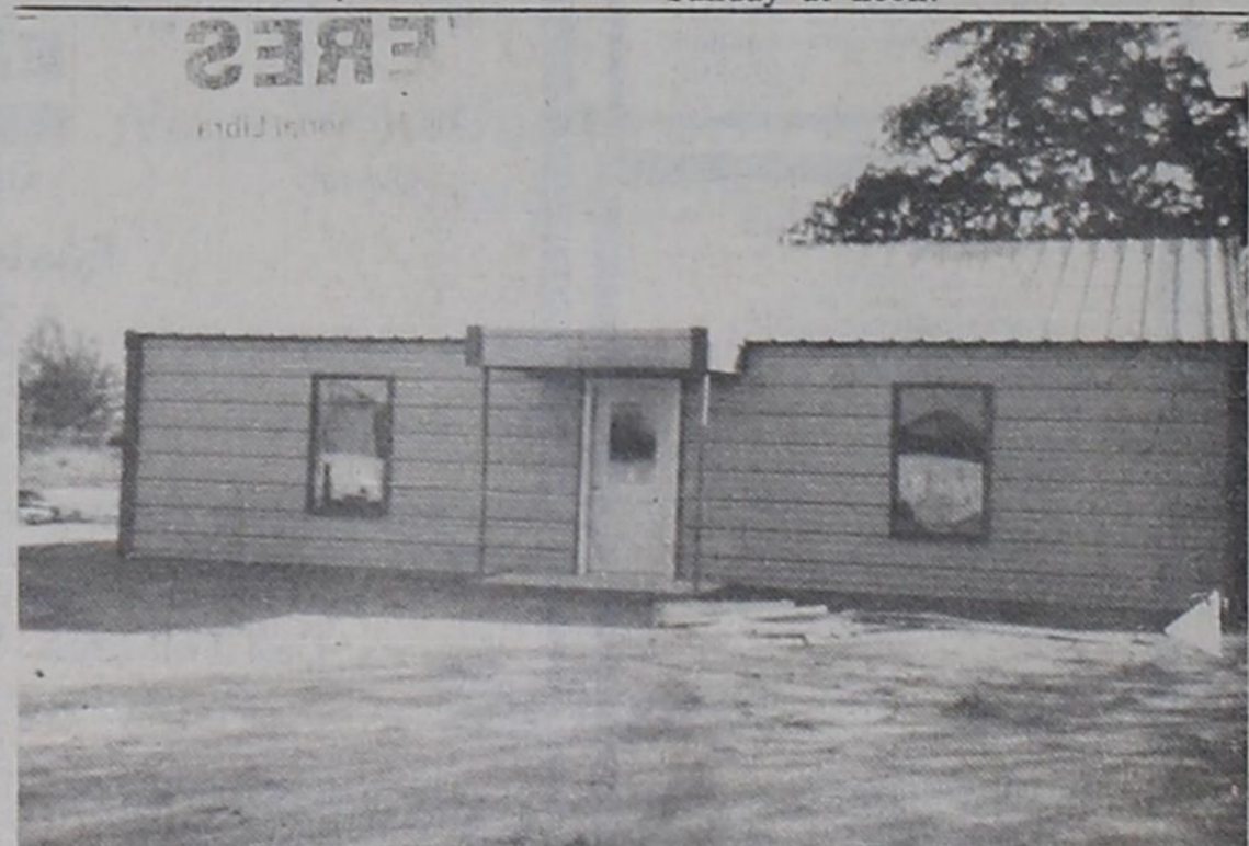
NEW CAFE BUILDING UNDER CONSTRUCTION — The building shown above is the new cafe being built by Carl Dean and Bertie Stacy. The building is located on east Hwy. 6. The exterior of the building has been completed and work is progressing on the interior. An opening date is expected soon.
