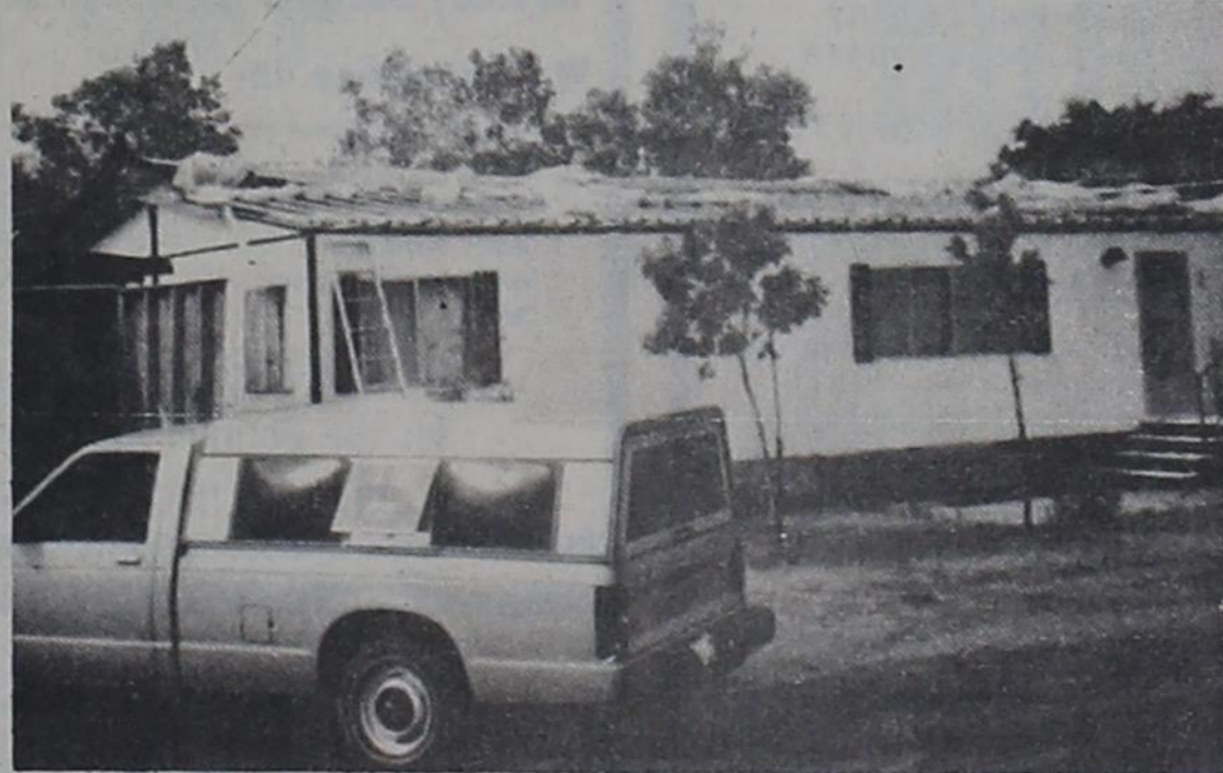
MOBILE HOME DAMAGED — The mobile home of William Isbell located north of town on Desdemona highway received heavy damage to the roof and interior from the storm clouds on Thursday.
