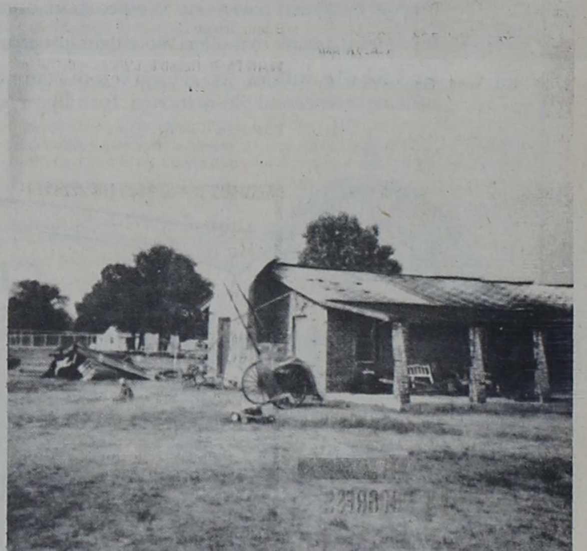
SHEET METAL ROOF DAMAGE - The sheet metal roof on Vernon Ables rent house was damaged during the storm. The front porch and the front half of the roof was peeled off.
