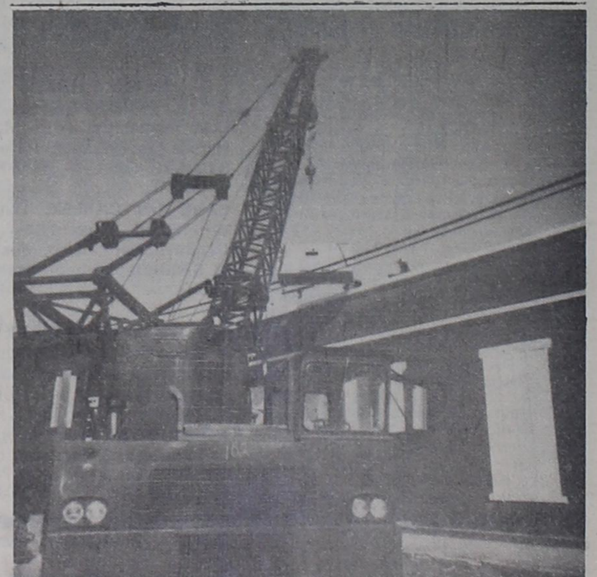
EAST END CO-OP GETS NEW HEATING - COOLING UNIT - East End Co-Op installed a new heating and cooling unit on Saturday morning to replace the unit which was damaged by a fire recently. The unit was installed by J&J Air Conditioning of Eastland, with the help of a crane from Eastland.
