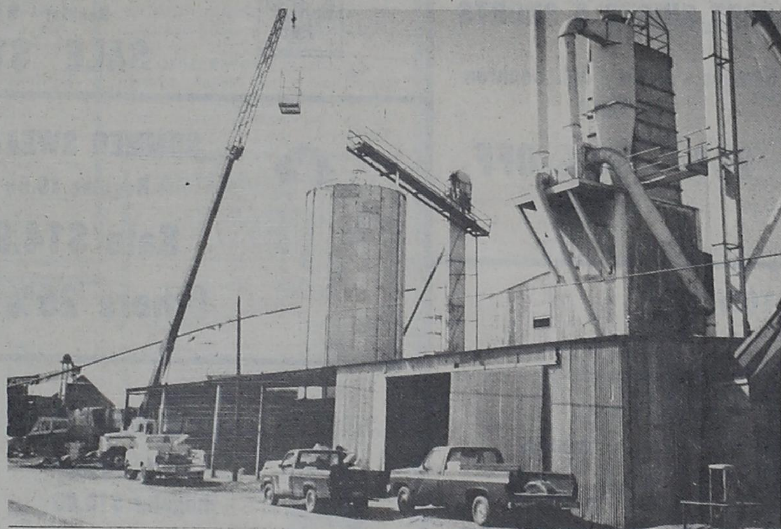
Shown is large Storage Tank recently erected at Gorman Milling Company.
