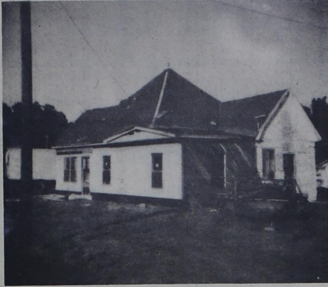
RENOVATING OF THE OLD LINDER HOME — Shown above is the progress being made on the renovating project by Mr. and Mrs. Jim Wood. That have made numerous changes throughout the home. The project is coming along fine.
