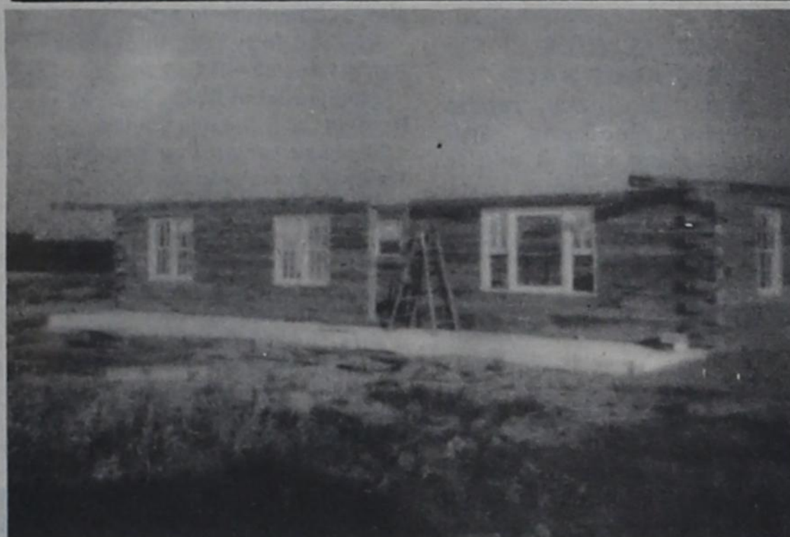
WORKING ON A NEW LOG CABIN — The picture above shows the new log cabin of Bill and Tammy Underwood with the side walls of the cabin nearing completion. The cabin is located in the New Hope Community.
