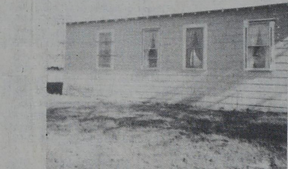
COMMUNITY CENTER DAMAGED — The Kokomo Community Center received broken windows and other hail damage.
