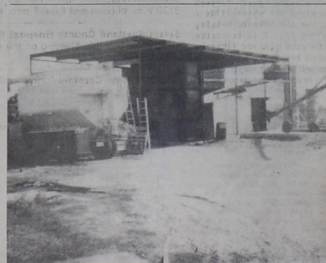
NEW CONSTRUCTION AT G&H FEEDS — New construction is being made at G&H Feeds located on Kokomo Hwy. north of Gorman. The firm has been in operation for past several weeks and have been trying to construct facilities at the plant site since its owners Bill Gressett and Daryl Hirst began the new business.
