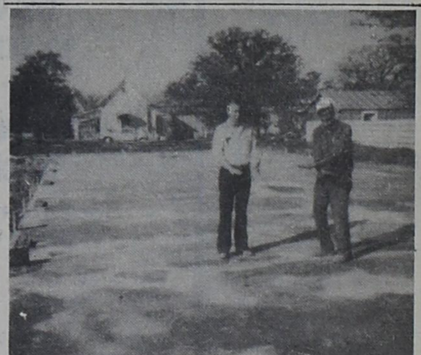
EVERYTHING CAME OUT SMOOTH — Gene Foster and Jack Harrison are shown putting the "smooth" whammie on the finished slab at the site of the new fire station.
