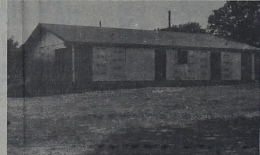
NEW HOME OF MR. AND MRS. RUSSELL CORDELL is shown above under construction on a track of land near Hi Point on the old Carbon Highway.
