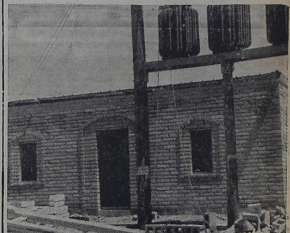
NEW OFFICE BUILDING AT BIRDSONG PEANUTS - Shown above is a portion of the new office building under construction at Birdsong Peanuts. This and other buildings under construction for the company are nearing completion.
