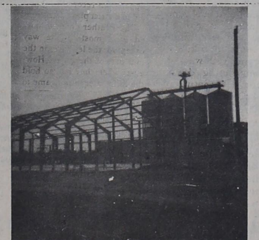
NEW EXPANSION AT BIRDSONG — This new building structure is being added in the vicinity of the new hull mill on the east end of Birdsong complex.
