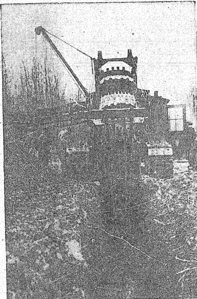
DIGGING THE "BIG DITCH" —A giant ditch-digger plows through Pennsylvania at a fast clip, taking everything in stride as it lays an oil pipe line to Northern cities from Texas oil fields.
