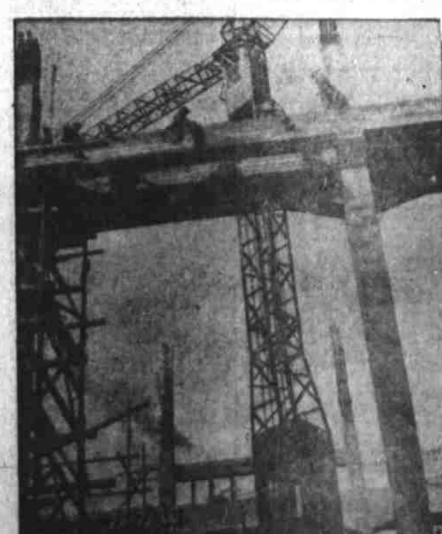
NEAR LIEGE, Belgium, stands a brand new power station which will increase the electricity output of both Belgium and Luxembourg. The power plant was partially financed through a loan of the International Bank for Reconstruction and Development.
