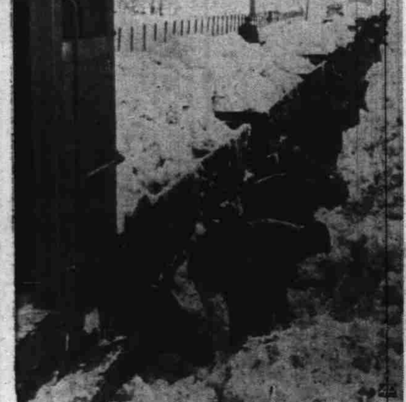
SNOW TRAIN IN ENGLAND — Workmen shovel snow from British railroad right-of-way onto coal cars which will dump it in valleys along the line. The snow is being removed to avert slides onto the tracks and flooding when a thaw comes. (AP Wirephoto).
