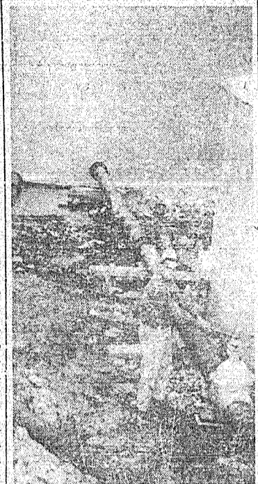
Pictured above is Clifford Stephenson turning the valve to let water into the new 500,000 gallon storage tank on the top of East Santa Anna Mountain. The valve was opened Wednesday afternoon of last week and by Thursday night had more than 300,000 gallons of water in it.
