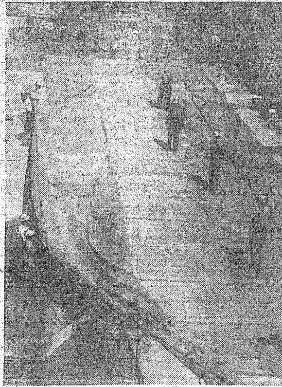
ROLLING OUT THE CARPET —Sixty feet below the surface of the ground in downtown Houston, workers stretch out a Butyl rubber carpet on which the 44-story Humble Oil & Refining Company building will stand when completed in 1962. The Butyl membrane will act as a water barrier for the foundation of the building. This is a unique application of the durable, flexible synthetic which is produced at Humble's Baytown Refinery and is widely used in everything from hot water bottles to conveyor belts, tubing, tires, wading pools, protective clothing for missile launching crews, and car accessories.
