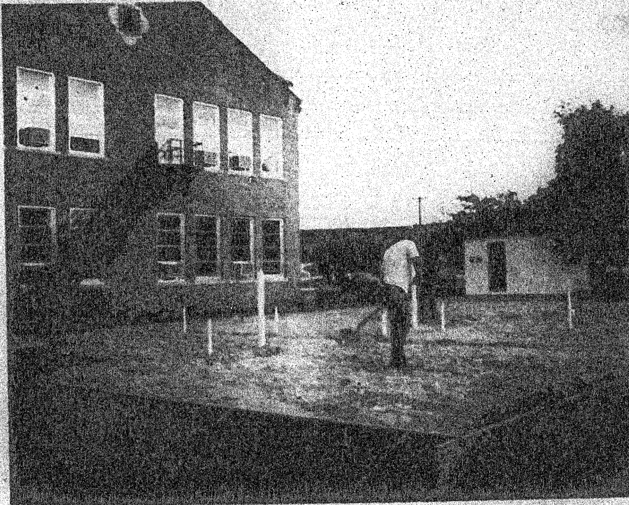
CONSTRUCTION STARTED... The new homemaking building at Santa Anna High School has been started by Davis Construction Company of Coleman. The building is located at the east end of the high school building and will be a modern
